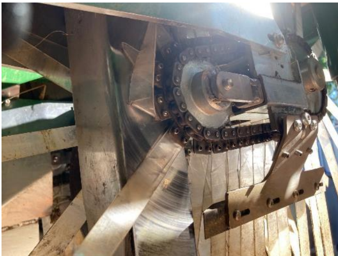
Blockage due to stuck slat
